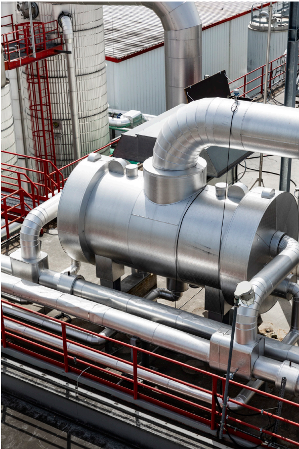
Installed on the roof, the Vahterus steam generator recovers heat energy from ethanol vapour to generate low pressure steam, which is the energy source for Pannonia Bio's stillage evaporation system.
