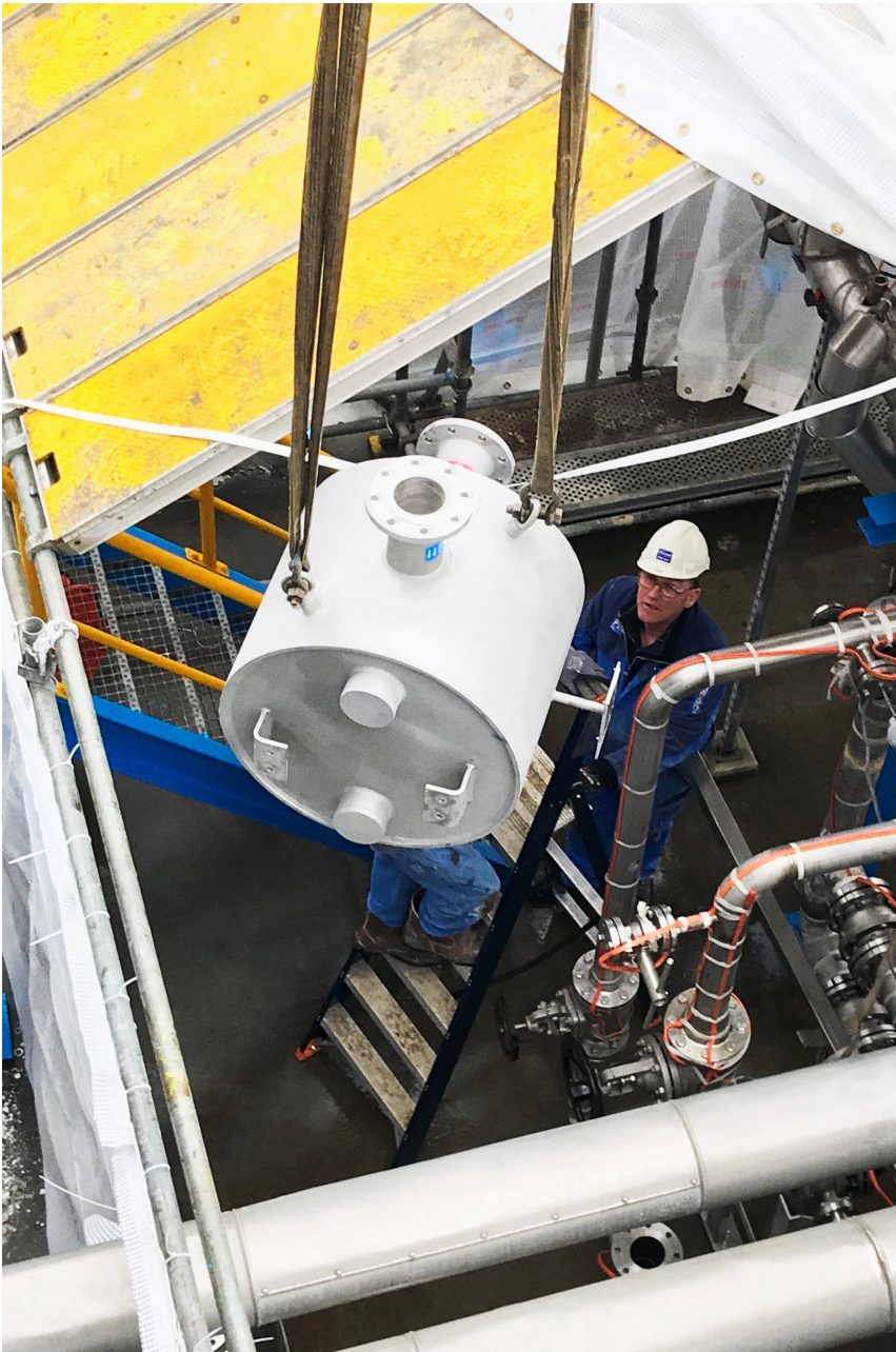
Installing the Vahterus PSHEs at Kisuma Plant required special arrangements.
