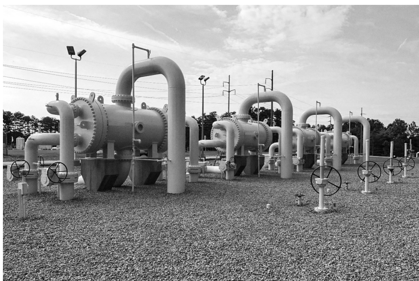
Vahterus heat exchangers successfully installed and running as per the customer requirements with operational performance data matching the design.
