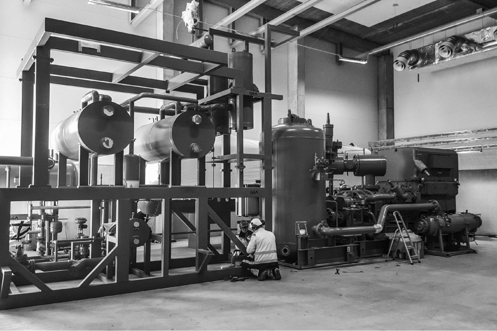
E.ON installation of four GEA heat pumps next to the sewage treatment and waste incinerator plant in Malmö, Sweden. The heat-pump system draws nearly 30 MW of heat from the sewage water Malmö's harbour area.
